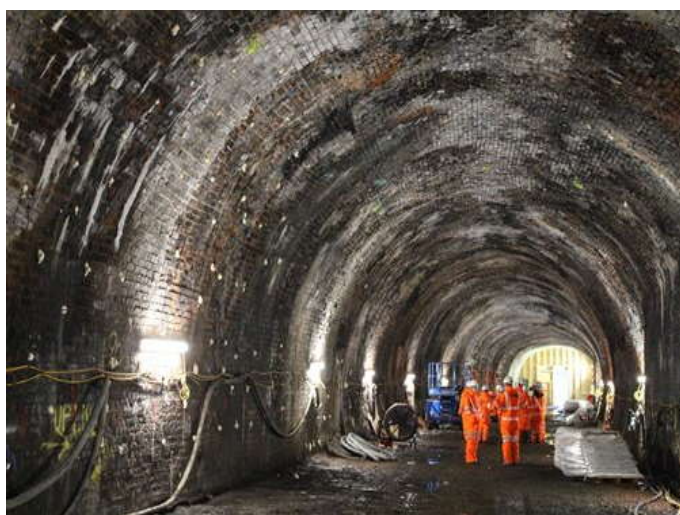
Install of Build Mesh CF 40020 For Reducing of Micro Concrete or Micro grout or Shotcrete Thickness, it from 150mm reduced until 45mm Thick
