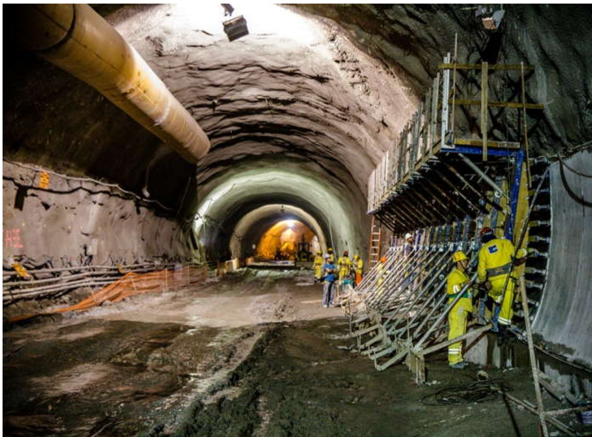
Install of Build Mesh CF 40020 For Reducing of Micro Concrete or Microgrout or Shotcrete Thickness, it from 150mm reduced until 45mm Thick
